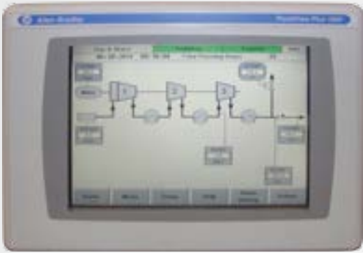
Allen Bradley PLC-based control center with PanelView Plus 1000 interface
