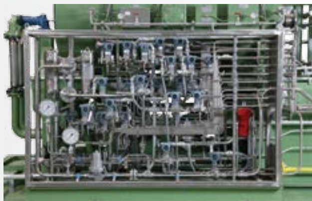
Gas seal instrumentation rack with 2-of-3 voting, seal and purge gas filtering
