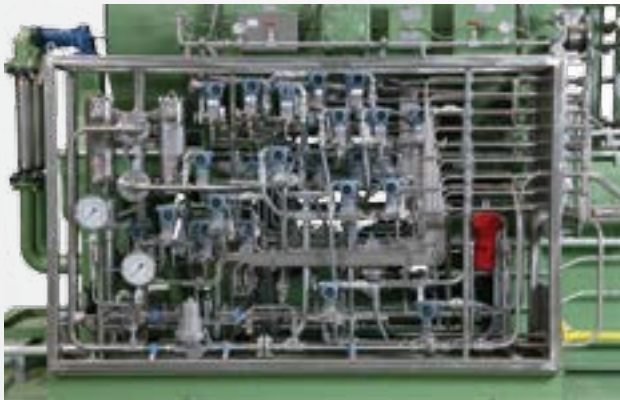
Gas seal instrumentation rack with 2-of-3 voting, seal and purge gas filtering
