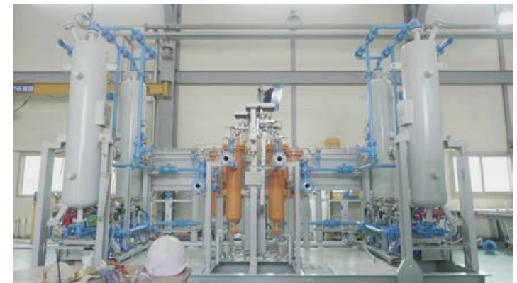
These compressor and dryer packages were built according to API specifications
